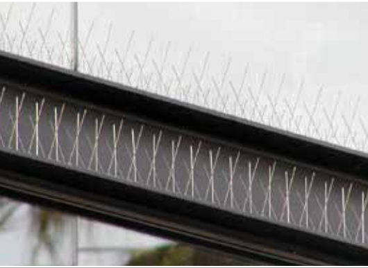
Multiple rows of Bird-Flite protect a steel beam from pigeons.
