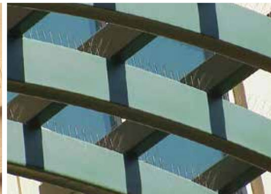
This attractive structure is protected against pigeons by Bird-Flite spikes.
