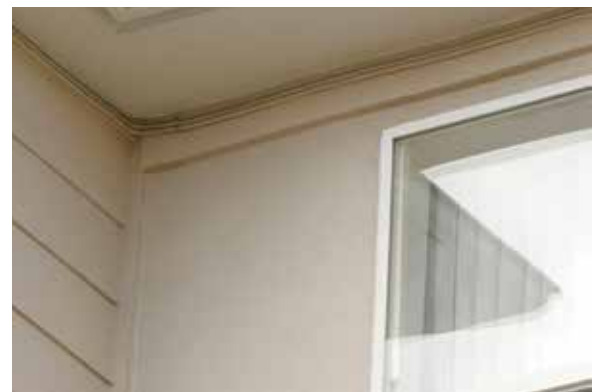
Bird-Shock Flex-Track installed under the soffit for mud swallows. One zap and they're gone for good.
