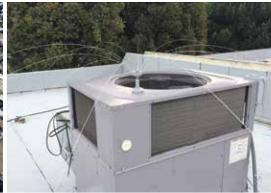
An eight foot Daddi Long Legs with magnetic base protects this large HVAC unit.
